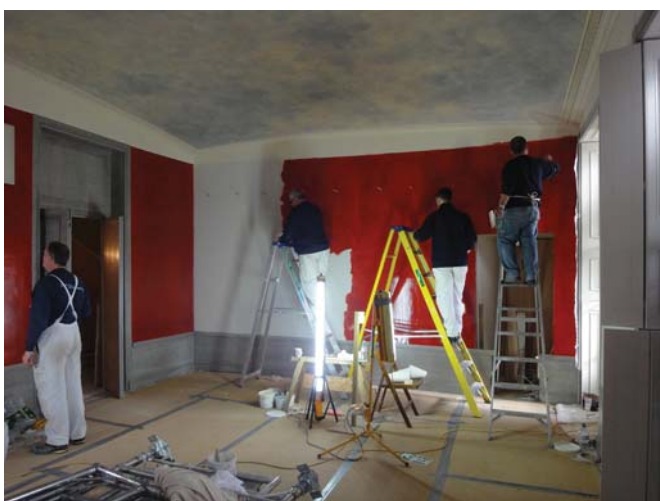
Work being carried out by by specialist painters from Hare and Humphreys Ltd to carefully recreate the Pompeian red and harewood decorative scheme in the first-floor Drawing Room – now the Exhibition Gallery – which has been restored to its original 1792 appearance based on research carried out by historic paint consultant, Helen Hughes. Photograph: John Bridges
