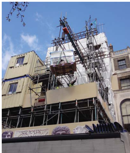
An exhibition case is carefully lifted by crane into the first floor of No.12. Photograph: John Bridges
