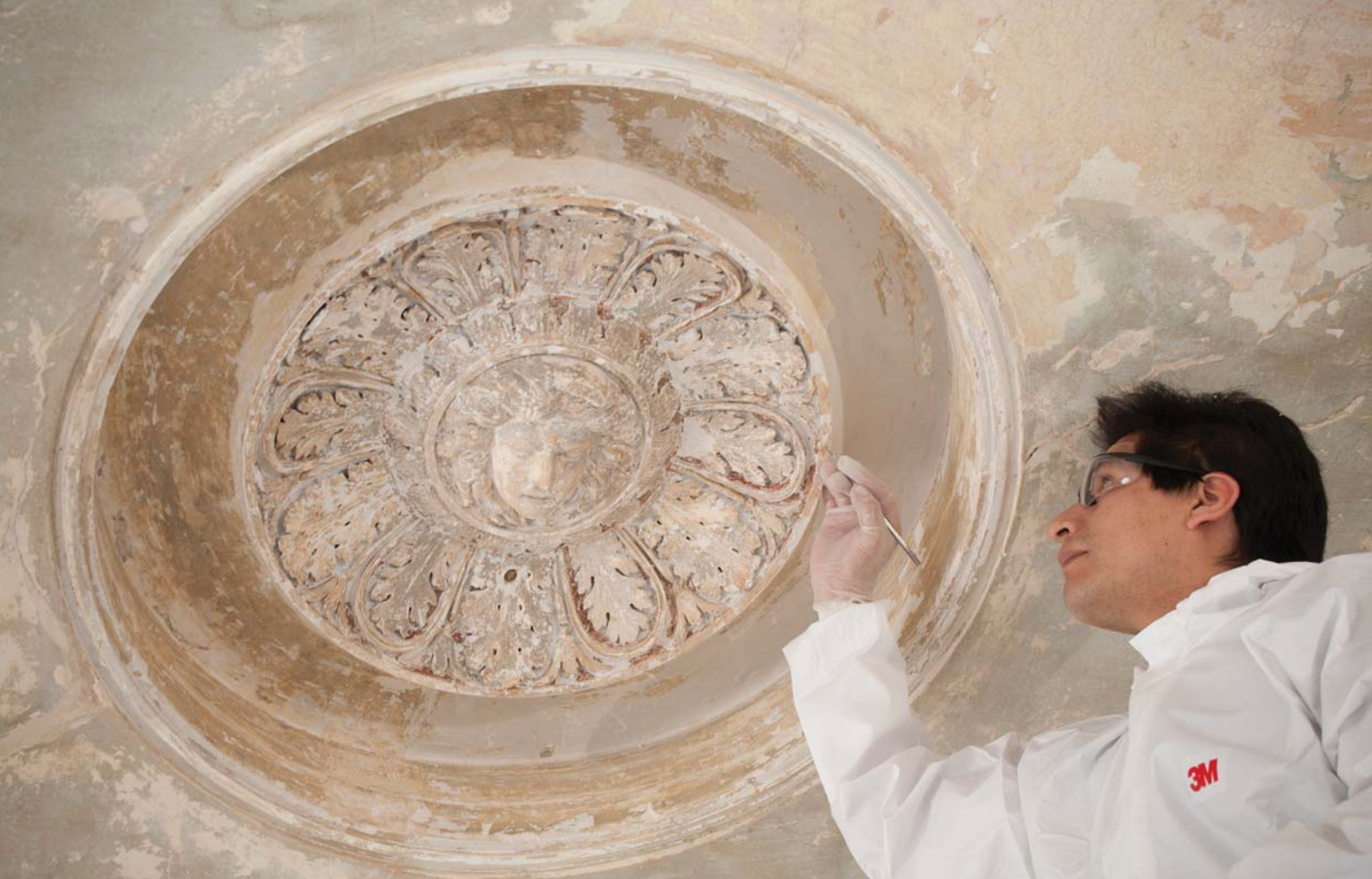
Exploratory work being carried out to the central boss on the ceiling of the first floor of No.12. Photograph: Ralph Hodgson
