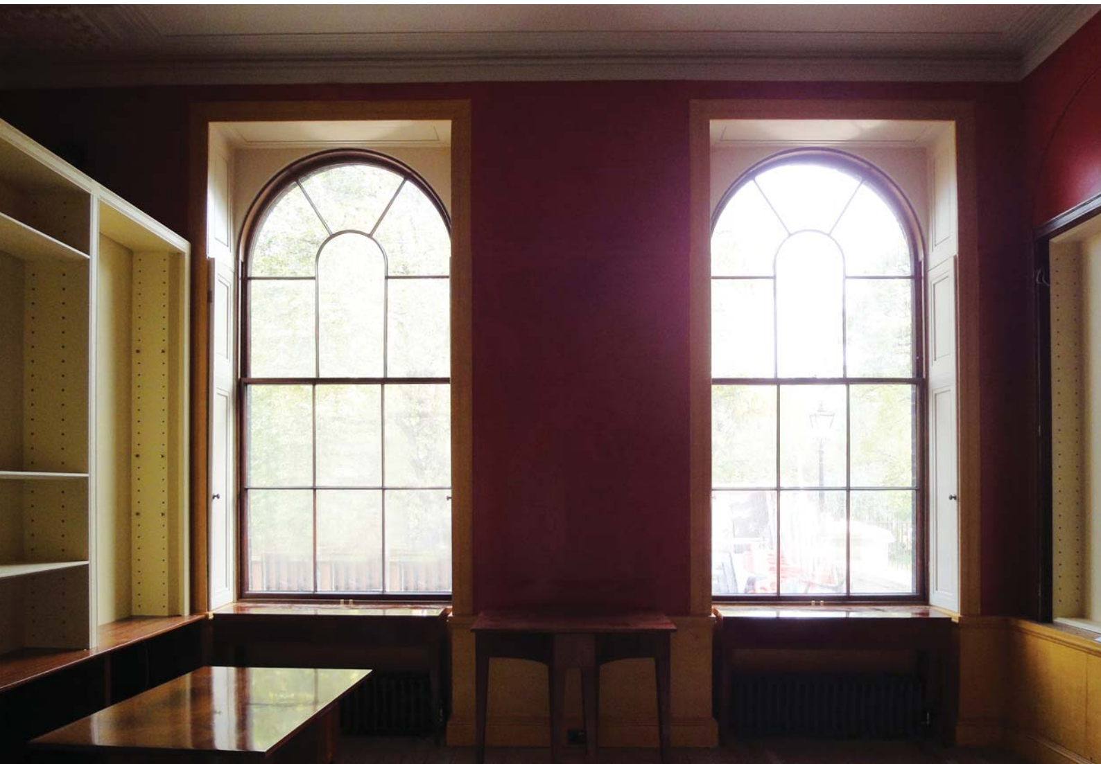
The ground-floor shop in No.12 in course of installation. Photograph: Lewis Bush
